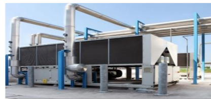
AHU Units & AC Ducts Spray- Dose:5%
